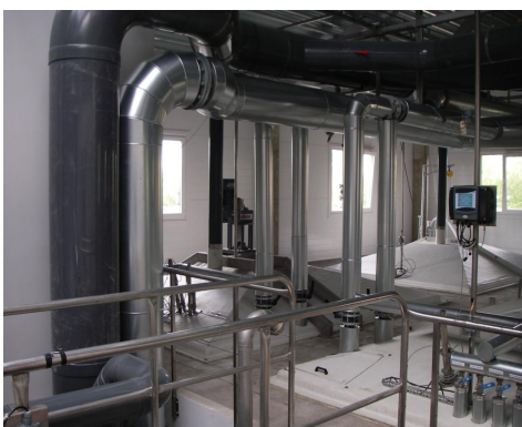
Covered MBBR reactors.
